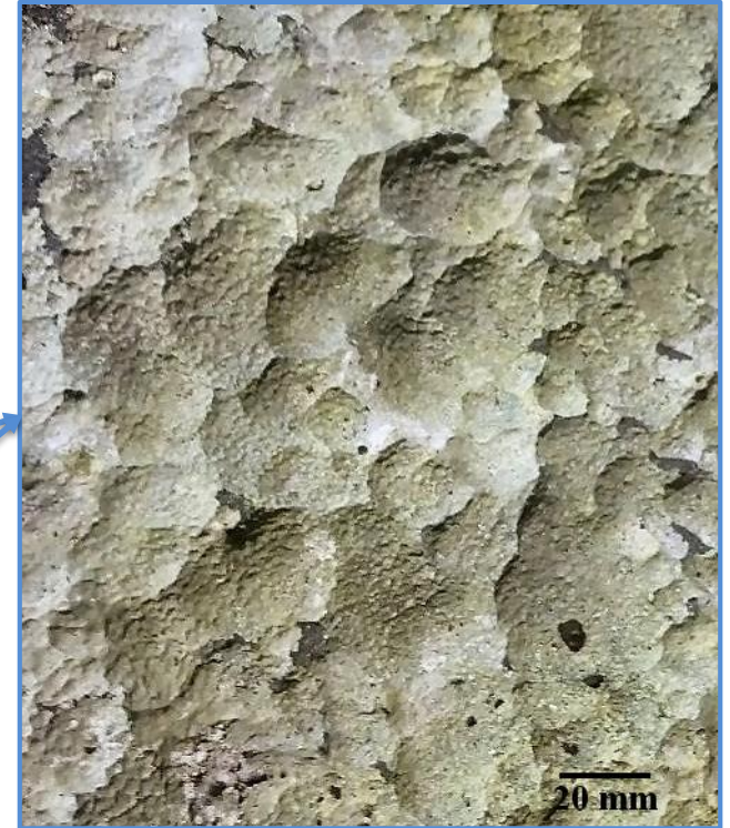
Pothole location characterized by pitting
